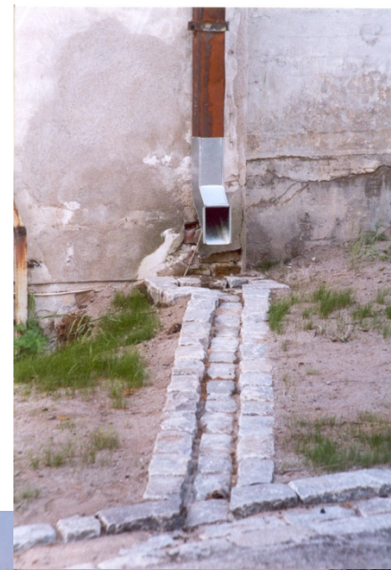
Disconnected roof water
