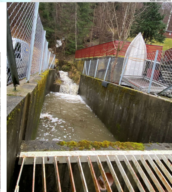
Drainage system with self cleaning grates
